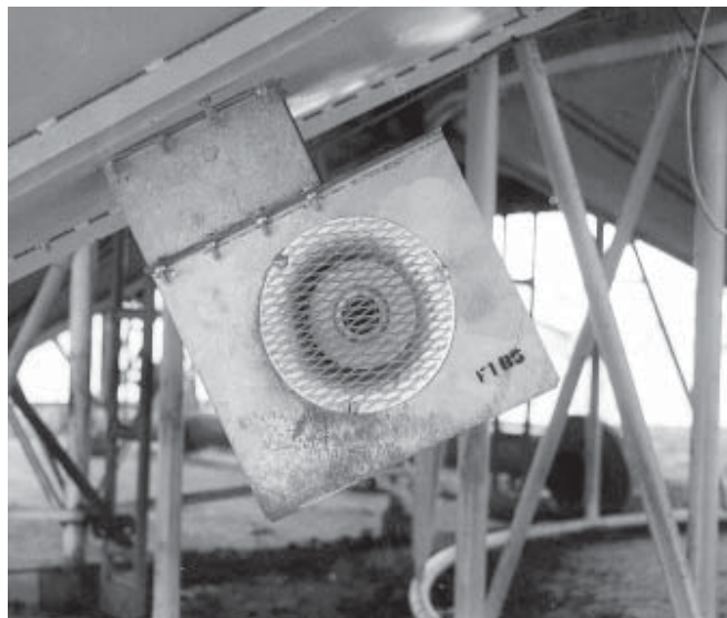
This simple aeration system with internal ducting and an inexpensive time switch is ideal to ensure safe storage of all grains.
