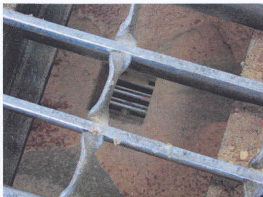
Figure 3.9 Top view of a receival hopper at SACBH showing the tubes of the magnetic separator.
