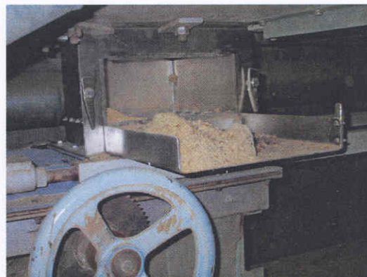
Figure 3.10 View of the frame of the magnetic separator under a receival hopper at SACBH.
